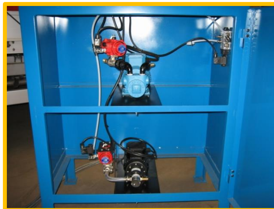
Typical Furan pump pack (2 pump system)
